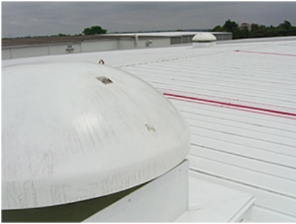
Electric rooftop exhaust fans for heat discharge
